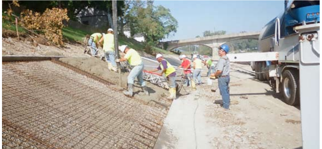
NEW CONCRETE REVETMENT BEING POURED IN TROY AS PART OF THE DAM SAFETY INITIATIVE.
